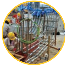
Acquired OHM Engineering to provide E&I Services
